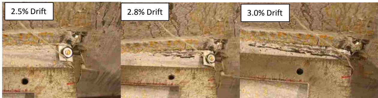
Figure 4.18: Crack propagation in N toe of mid-span gusset-to-beam weld (WT1,2).
