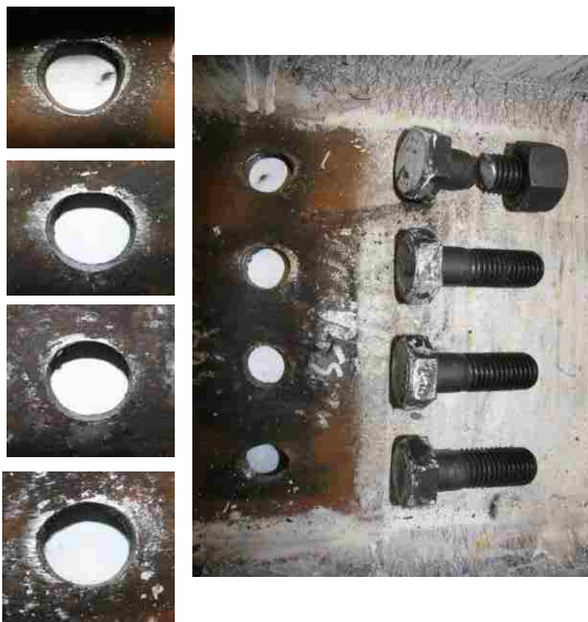
Figure 4.28: S beam web bolt hole elongation.
