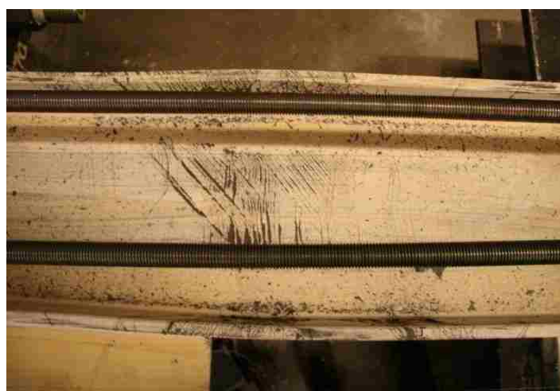
Figure 4.74: Initial S col. local buckling at +2.2% drift (LB1-IF/OF).
