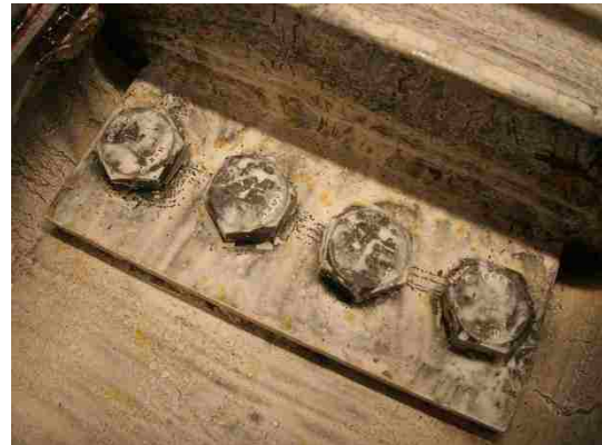
Figure 4.10: Initial shear tab yielding at -1.1\% drift (Y1).
