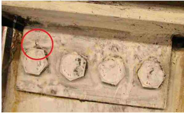
Figure 4.33: Initial yielding in N shear tab at +0.4% drift (Y1).
